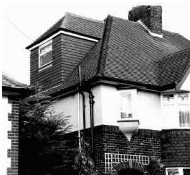
An unacceptable bulky dormer
