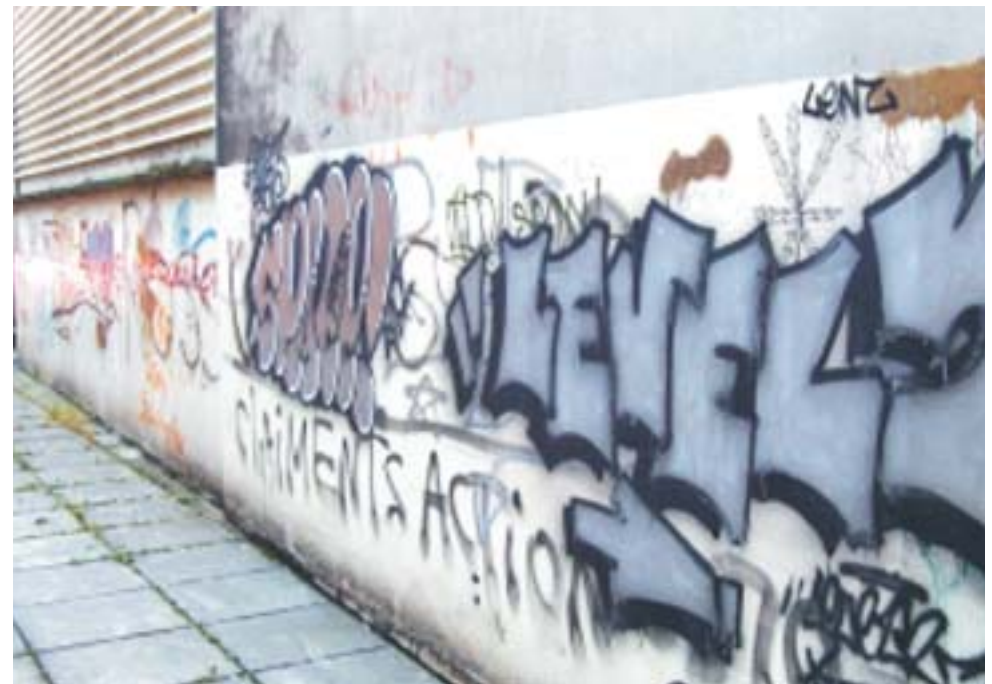
Inactive edges and poor maintenance of this area has resulted in this wall becoming increasingly problematic. If graffiti is not dealt swiftly others will quickly add to it.
