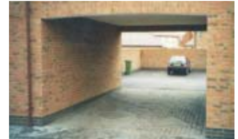
This parking court does not benefit from internal natural surveillance and the entrance is poorly defined. This clearly has the feeling of a parking area rather than a place in its own right. The paving is the same as that in the public area. This reduces the feeling of this being a private space and will not be as effective in deterring people who have no purpose in entering.
